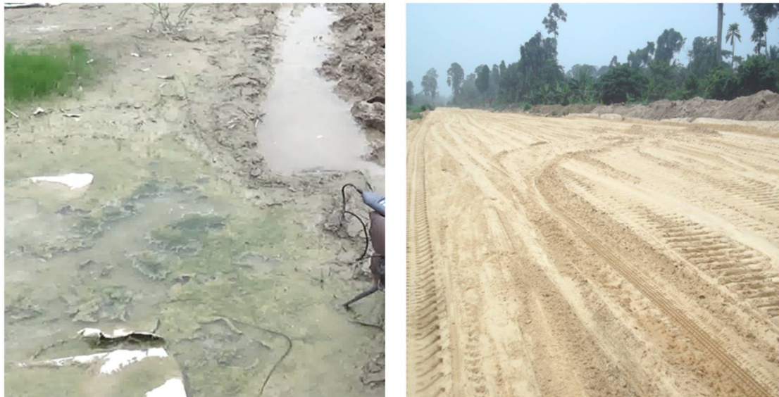
Figure 3: Site condition and construction practice in the Niger Delta - (a): Soft subgrade with puddle of water; (b): Sand filling to formation level
